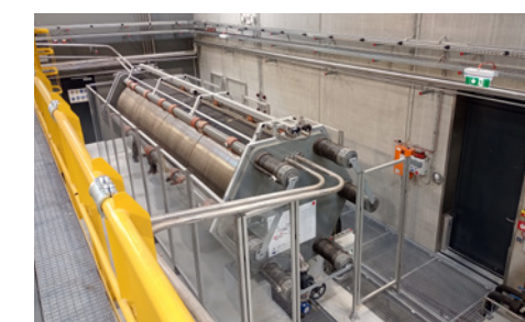
Demo4Grid Hydrogen Project, AUT
